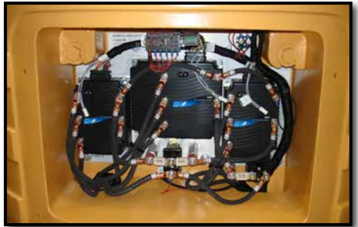
Rear Controller Compartment and Counterweight
